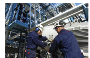
Heating & cooling Systems & Pipework
